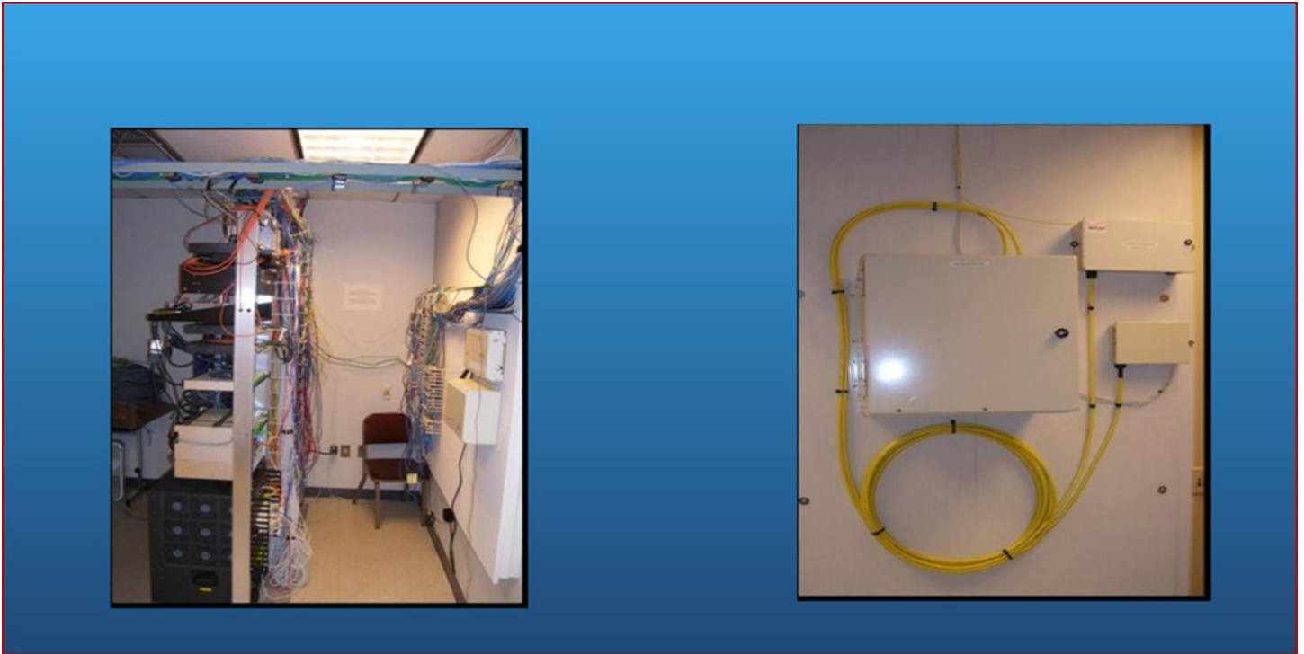
Figure 5 - Copper Infrastructure contrasted with Fiber Infrastructure
